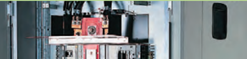
Power Conversion And Distribution
