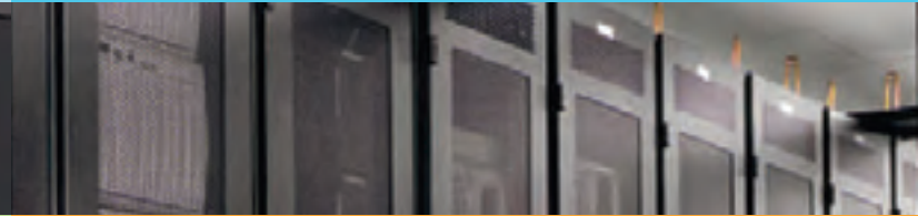
Integrated Racks And Cabinets
